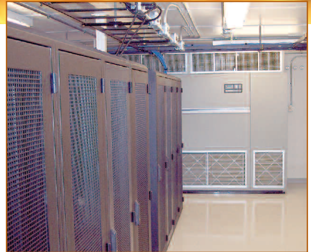
Server Vault with Liebert air conditioning system, "Unimount" track ceiling, and wire rails eliminate the need for raised flooring expenditures.
